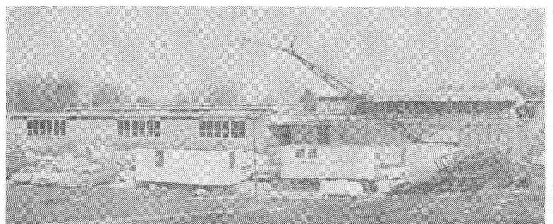
(Photos by C. B. Rainbolt, Jr.) THE ROAD TO SUCCESS — The scene above is the new grade school from a point northwest of the building. Below, construction from the south-east.
